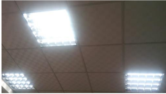
Example of Energy Efficient Appliances Usage: Use of LED lighting (Tanta University, Egypt)
