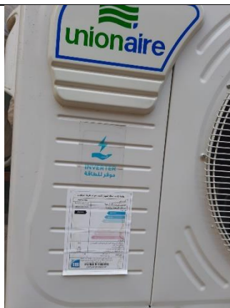
Example of Energy Efficient Air Conditioner (Tanta University, Egypt)
