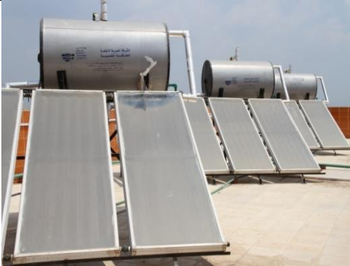
Solar Panel at student hostel (Tanta University, Egypt)
