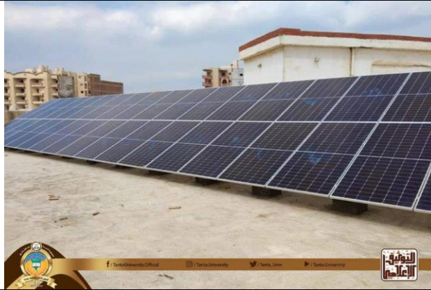
Solar Panel at faculty of Engineering (Tanta University, Egypt)
